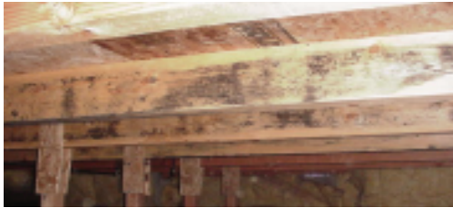
mold discovered after home occupancy
